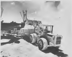
Slated sulfur poured from a payloador into a hopper mounted on the HDS pier conveyor system lands on the moving belt through an opening at the bottom of the hopper.
